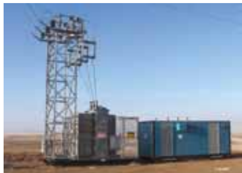
Surface Coal Mine, China – Substations
