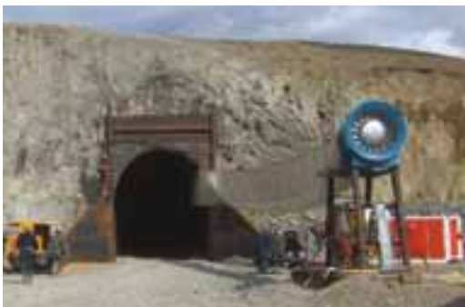
Underground Gold Mine, Russia – Moveable Substations
