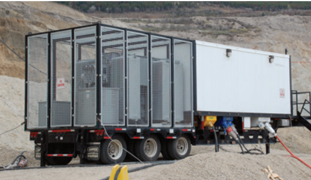
Open Pit Copper Mine, Canada – 13.8kV Mobile Substations
