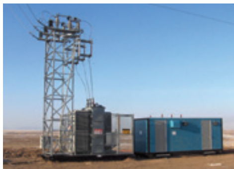
Surface Coal Mine, China – Substations
